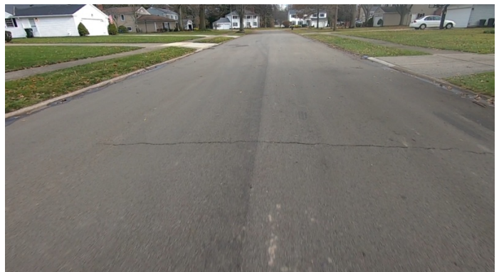
Upcoming Crack Seal Candidate
