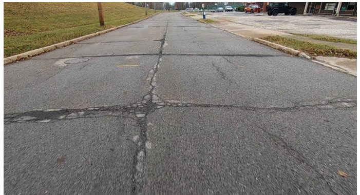
Roadway that Did NOT Receive a Crack Seal Treatment at the Right Time
